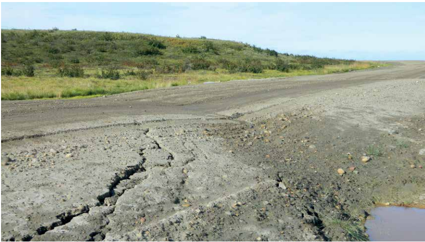
Dip in a road surface near Tuktoyaktuk, Northwest Territories. Only two weeks before this photograph was taken the road had been levelled. The subsidence is due to melting of ground ice below the road.
